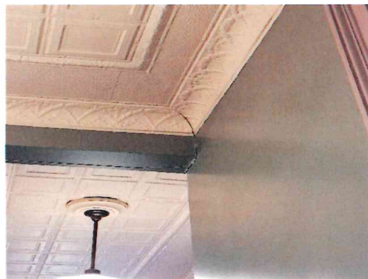
Cracking at Corner connections
