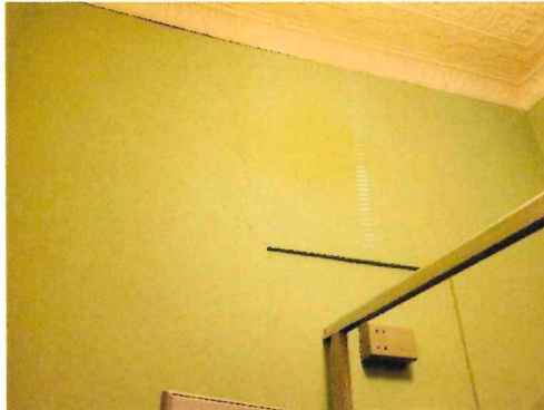
Men's Restroom cracking on east wall
